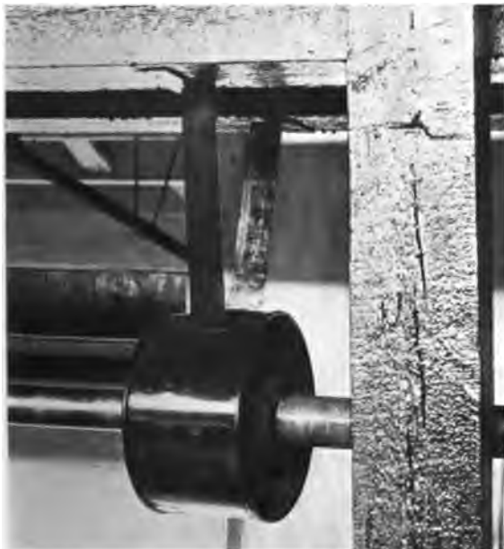
Fig. 6. Guard for Couplings already in Place.
